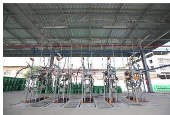
Exhibit 41: Gas filling plant
